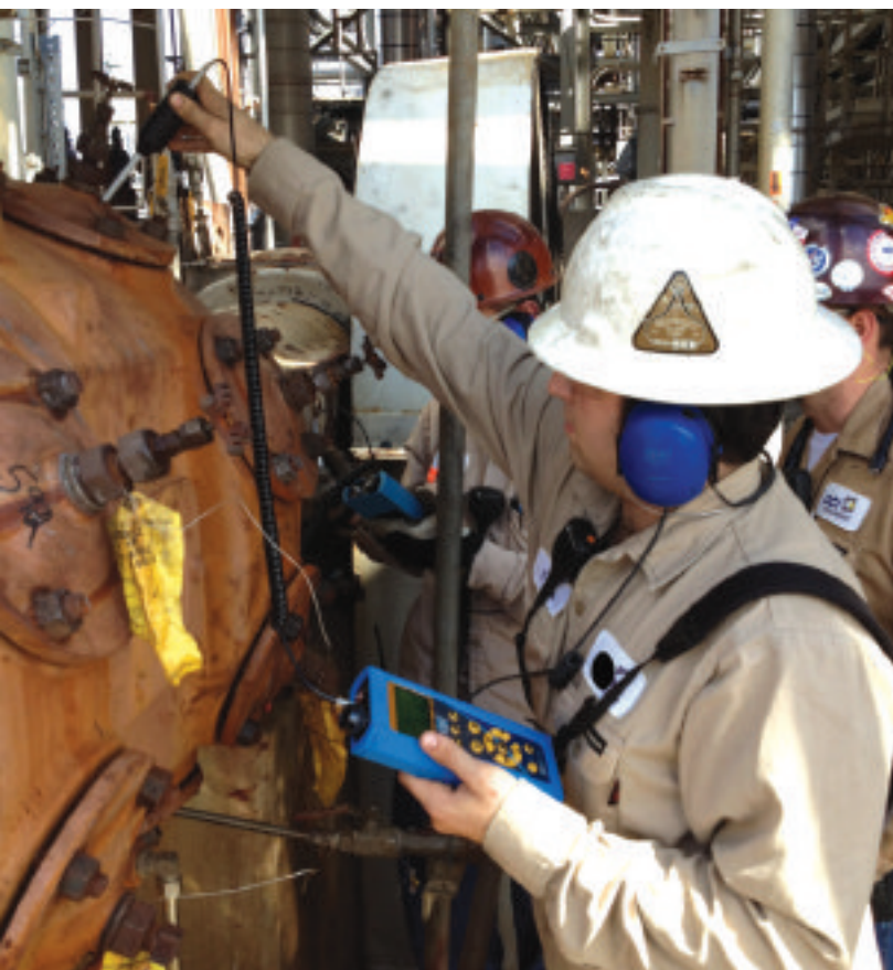
■ A technician uses an ultrasound needle sensor to test for problems.
