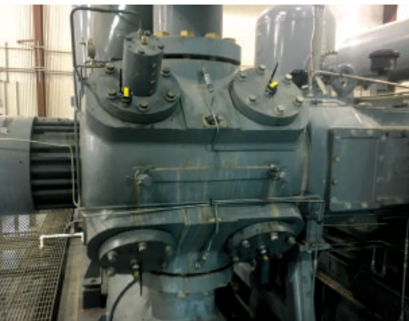
■ Vibration sensors with wireless transmitters are attached to the suction and discharge valve caps.
